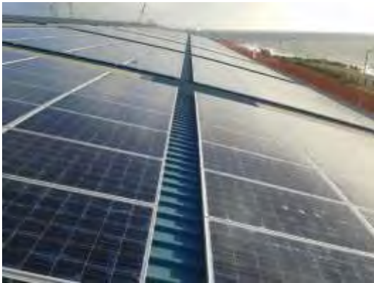
Solar panels on warehouse roofs
